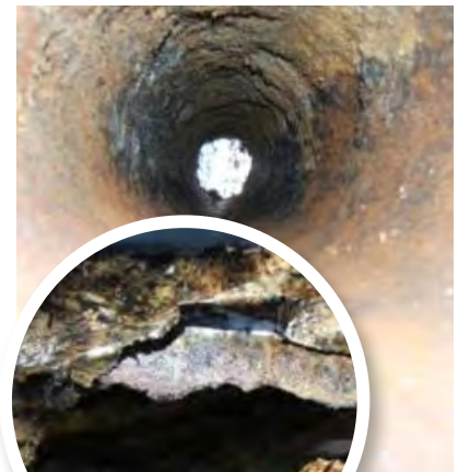
Corrosion in metal pipe wall
