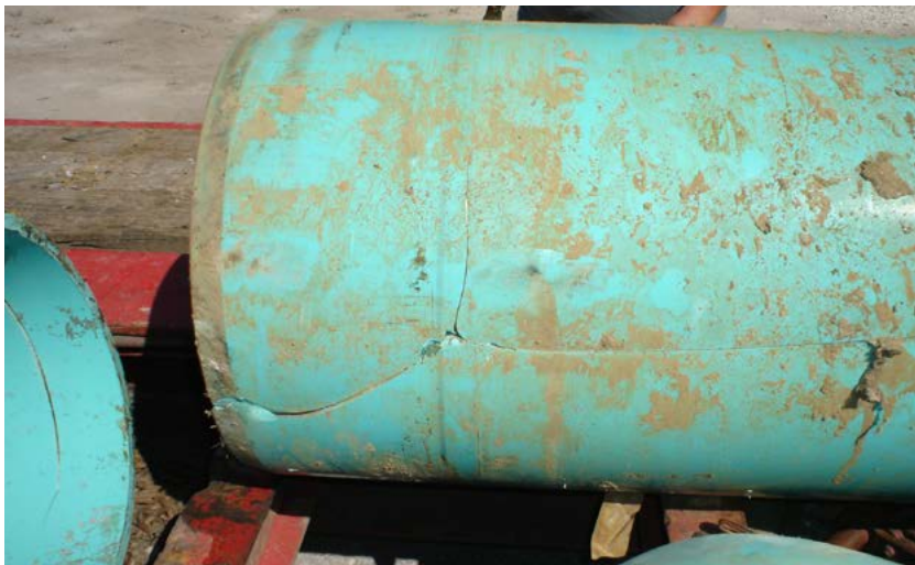
Broken PVC pipe
